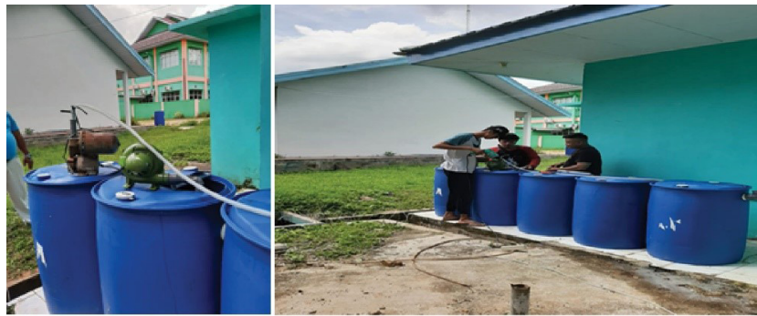
Figure 2. Blower and water pump
