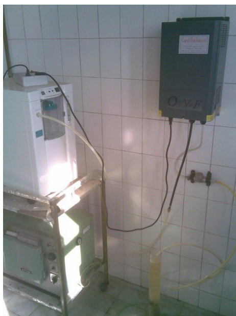
Figure 3. Ozone generator unit with generation power of 5 g/hr
